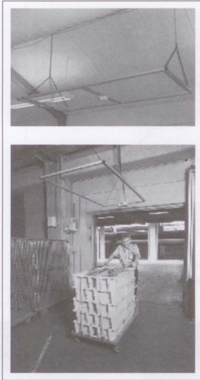
Figure 5 - Low-frequency antennas EH21 Exciter
